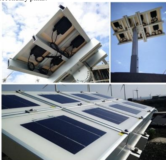
Figure 2: View of the support structure, showing the tilting head (up-left), exchangeable pillar (up-right) and mini-modules attached with clamps (down).
